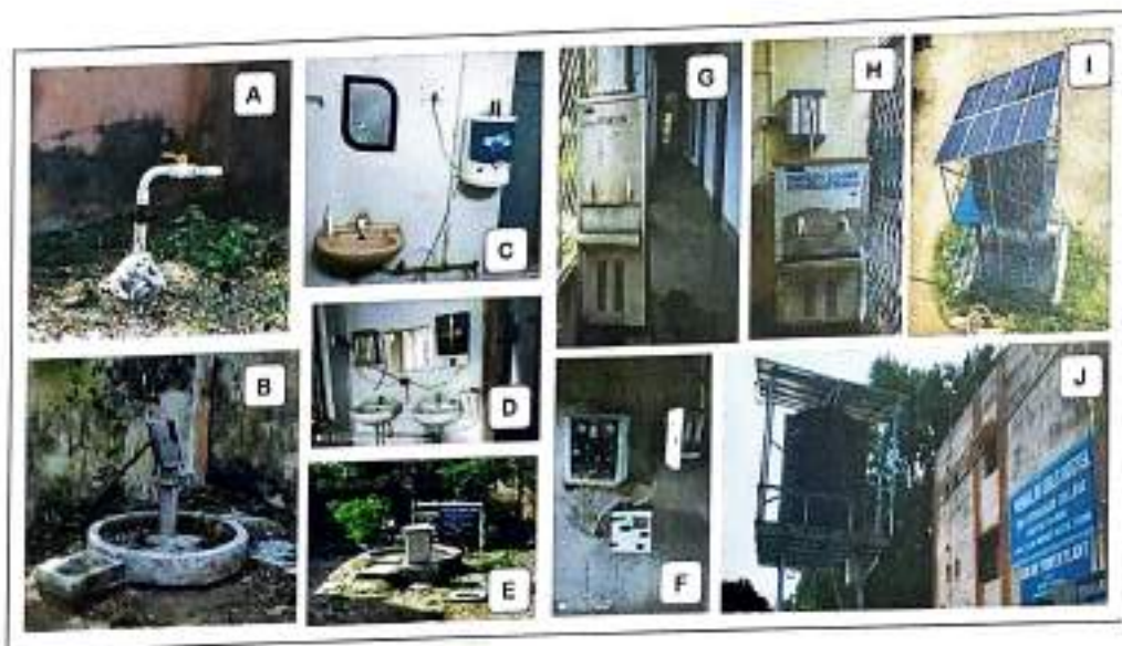
Fig. 1 : Drinking water facility of the College
