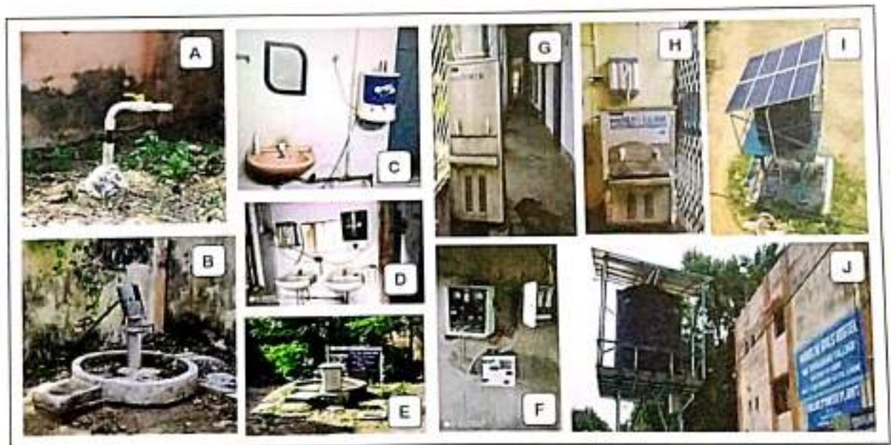
Fig. 1 : Drinking water facility of the College Campus
