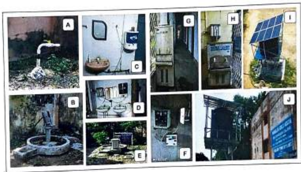
Fig. 2 : Drinking water facility of the College Campus
